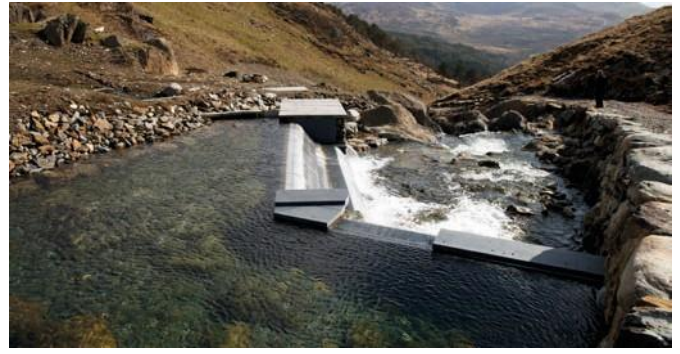
Hydro installation at Hafod Y Llan, one of the 8 hydros to date that generate 2,879,744 kWh of electricity
